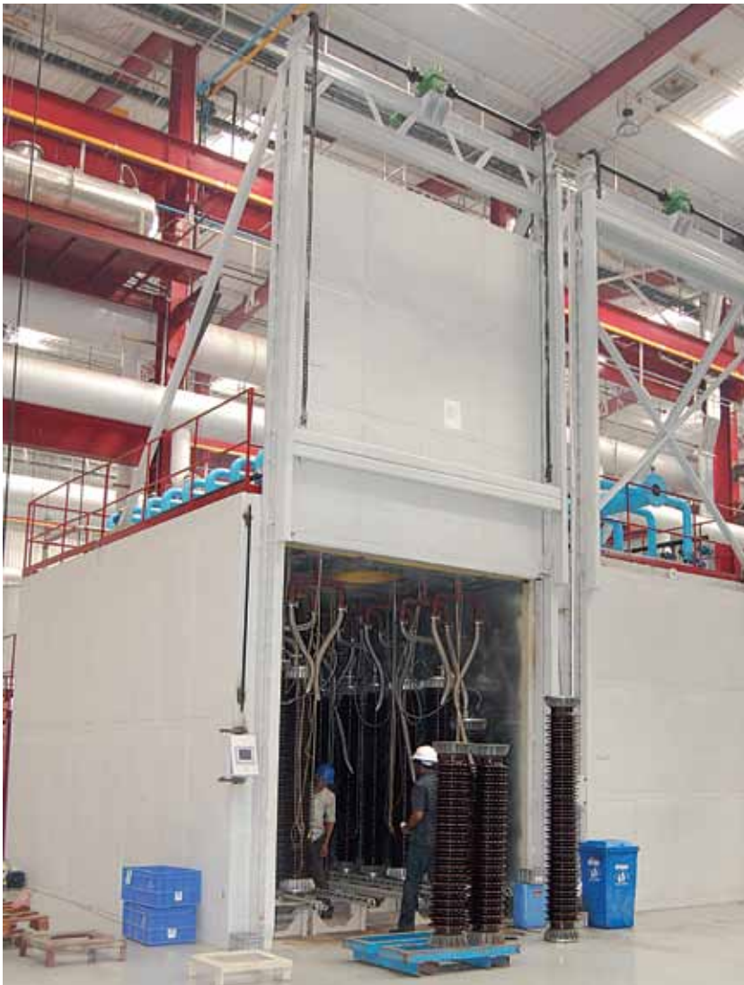
Transformer Drying Oven
